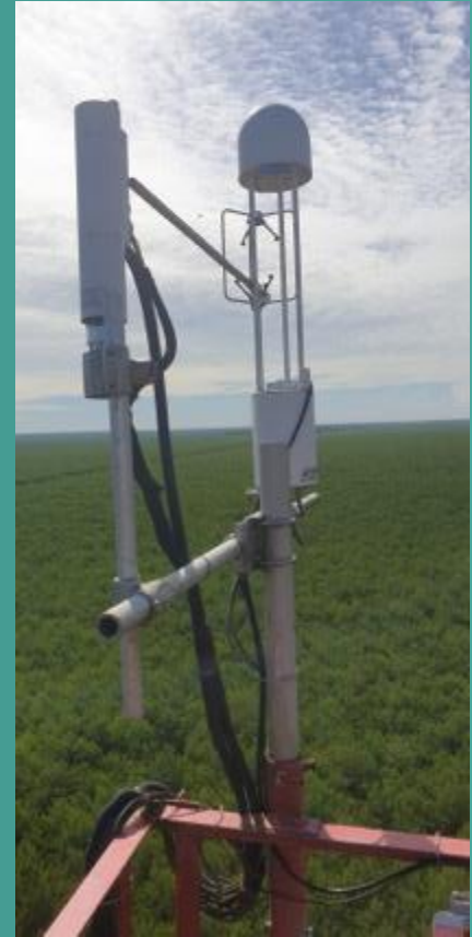
Tower for carbon flux measurements, APRIL planation, Kerinci, Riau Province, Sumatra
